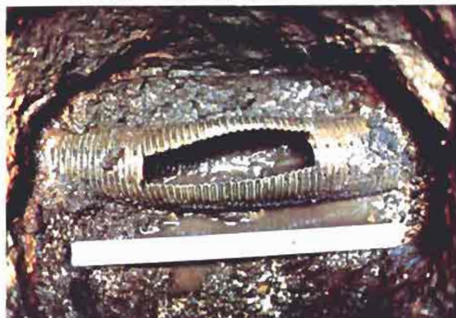
Coarse gravel, 5-30mm in size. Field drain Nr 16 Trial pit in field 12 II. June 1983
