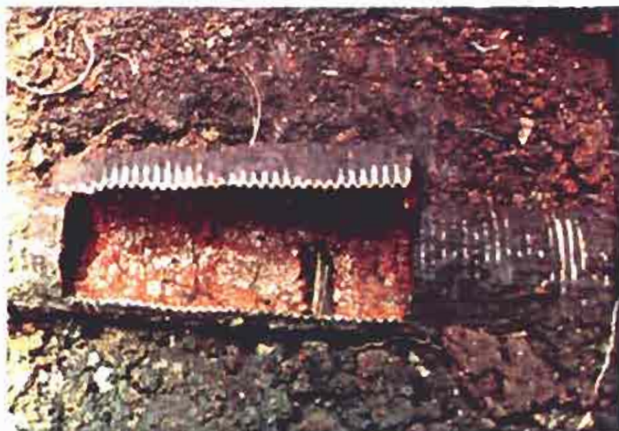
No surround other than loosely backfilled soil. Field drain Nr 4, Trial pit in field 12 II. June 1983
