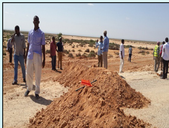
Field visit by participants to a section of the main road between Garowe and Dangaroyo damaged by floods in Puntland
