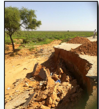
Damaged section of a road in Puntland
