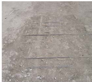
Parts of Barrage deck slab with Exposed Reinforcement steel
