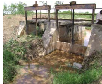
The off take structure of canal no 5 is in good condition but concrete is broken on the underside exposing the steel reinforcement, no gates and lifting mechanisms
