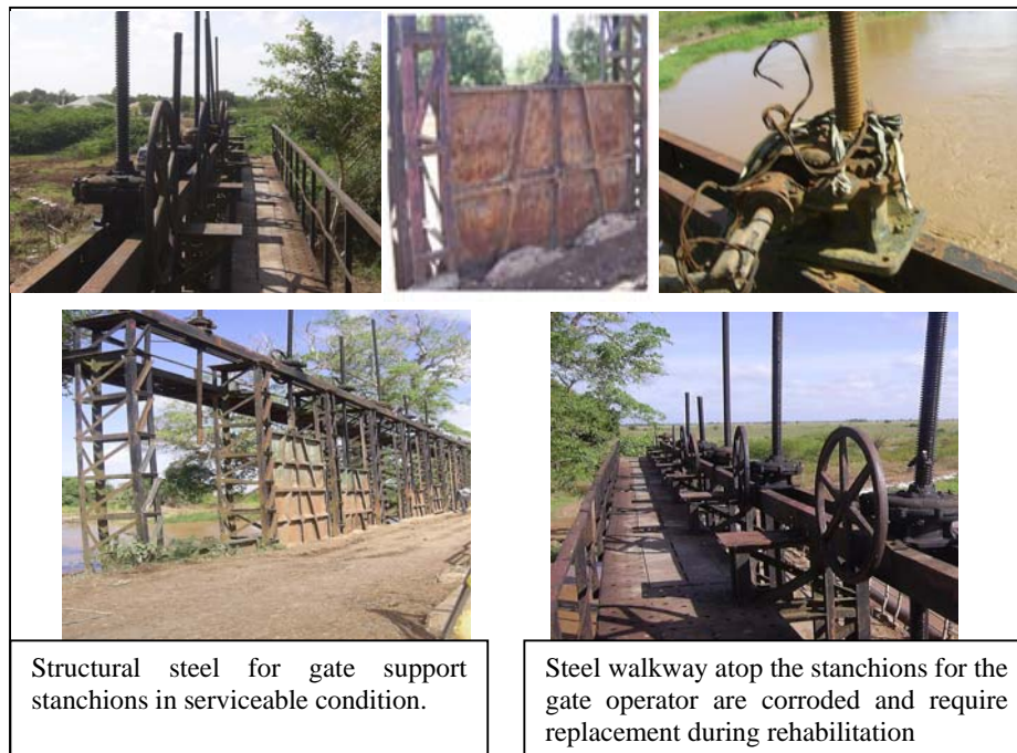
Figure 6.4: Status of gates, superstructure and lifting mechanisms in Qoryooley barrage
