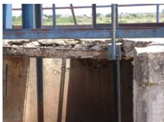
Exposed reinforcement of side Walk-way with loosely held Guard rails
