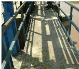
Side walk way with cracked concrete
